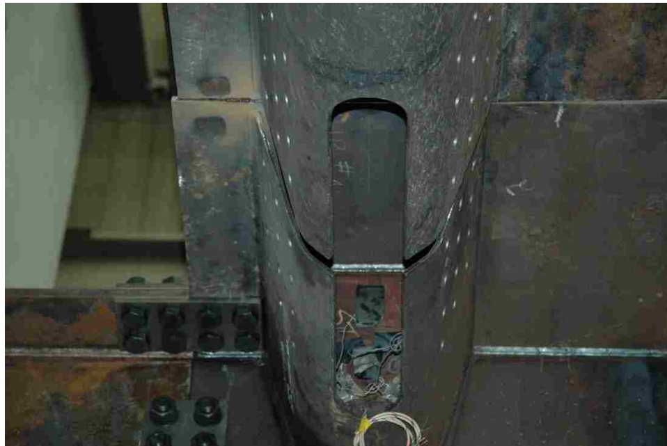
Figure 112 Lack of alignment of the ribs
