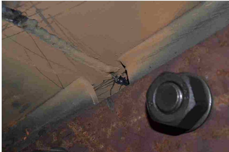
Figure 118 Lack of access over the rib wall for re-welding
